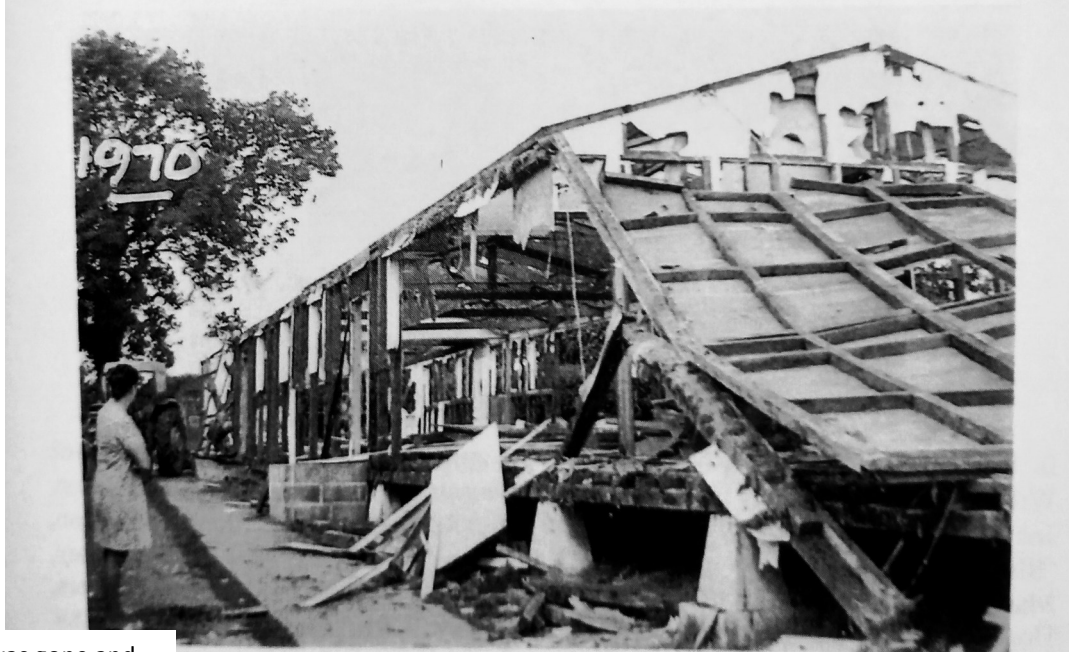
1970: The Village Institute being pulled down to make way for the new Village Hall
